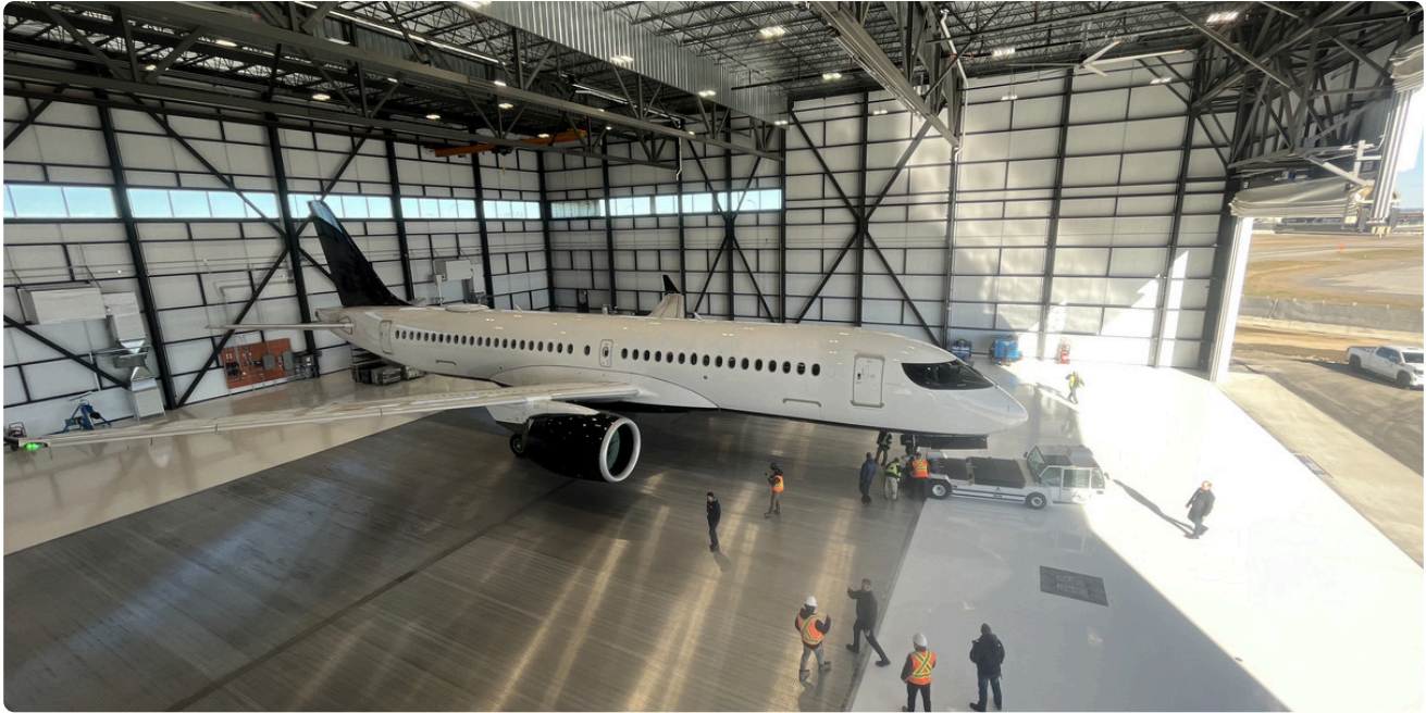
ILDFA installed and commissioned in a Airbus A320 4 bay hangar for Avianor, an MRO based in Mirabel, Canada
