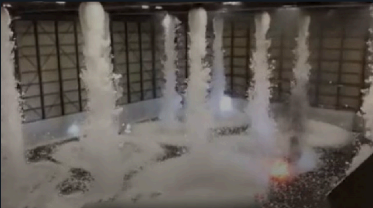
High Expansion Foam system commissioning at SFO, source: RJSD website
